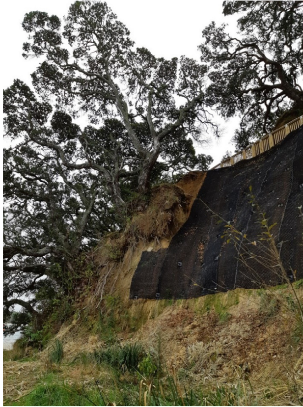
Photograph 1 - Photo of tree and exposed lower roots
